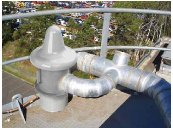
VHS Pressure Relief Valve releasing excess pressure
